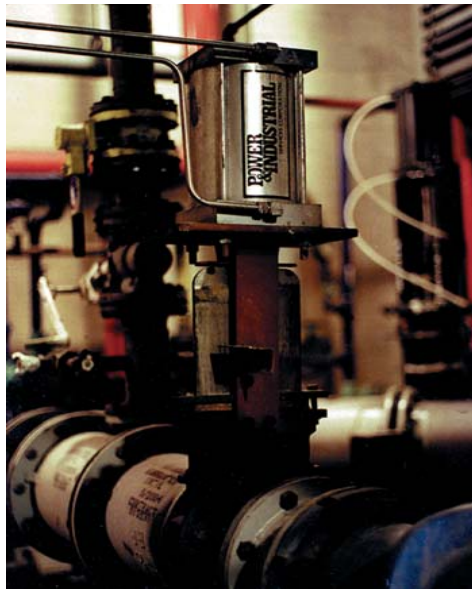
BOTTOM ASH SLURRY
